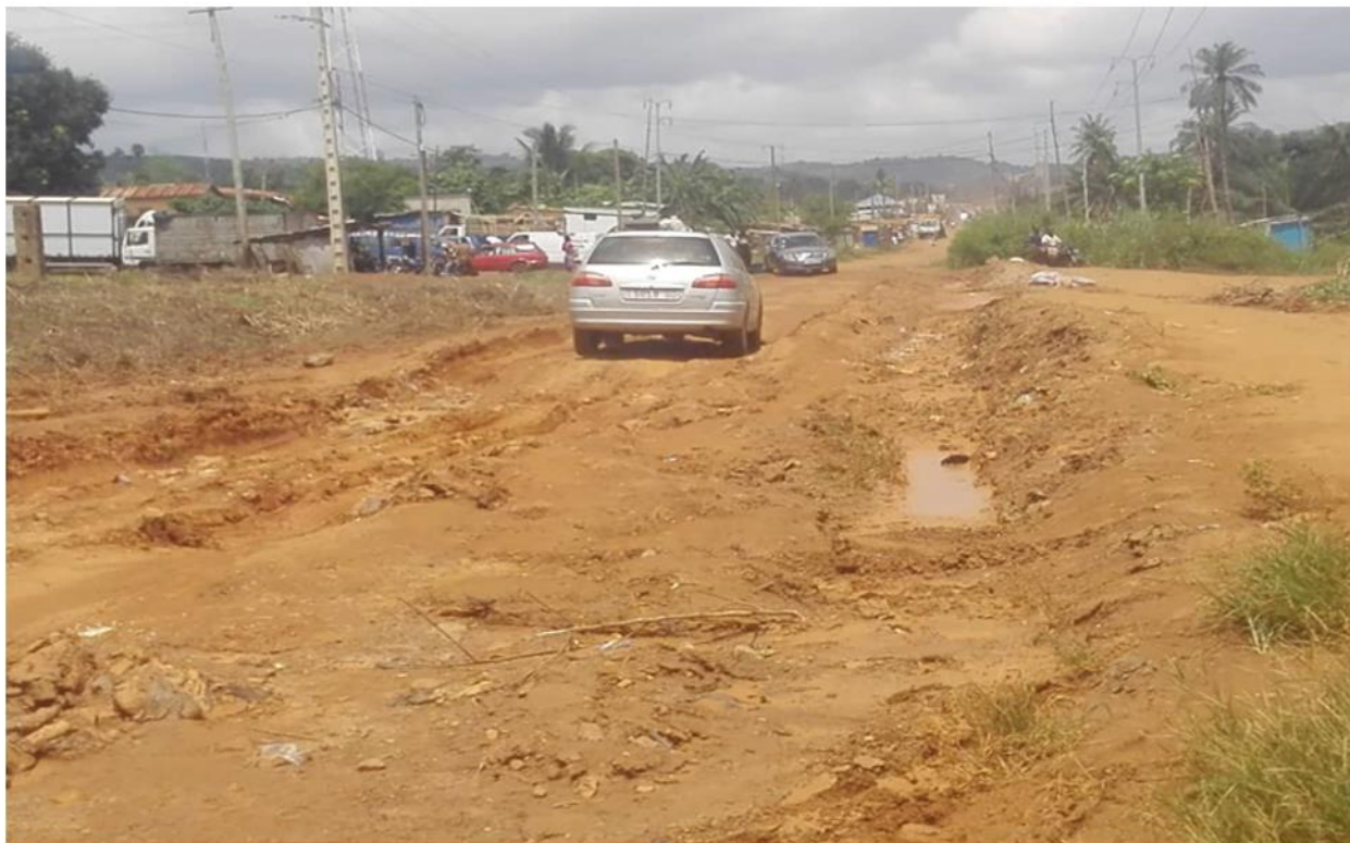
Figure 8. Degraded service road in Alinka (Agoè-Nyivé 4).
