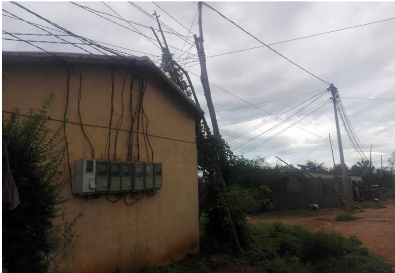
Figure 7. Spider web electrical connection at Akato (Gulf 7).
