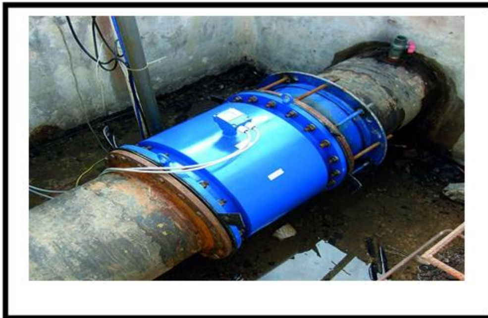
Figure 6. Permanent Flow meter [12].
