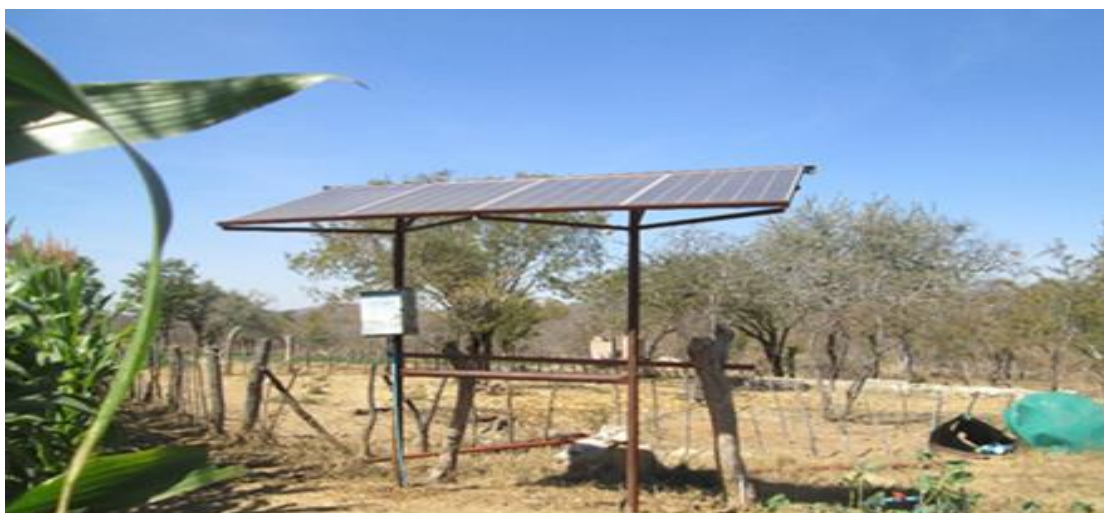
Figure 3. A submersible solar-powered borehole irrigation system in Matedza village.
