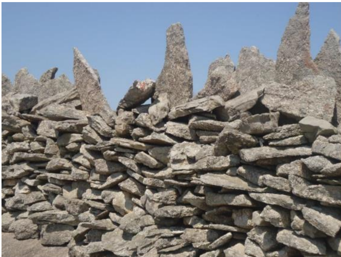
Figure 2: Section of dry stone wall at the Etoo site. Source: Labiyi Nestor, 2017.
